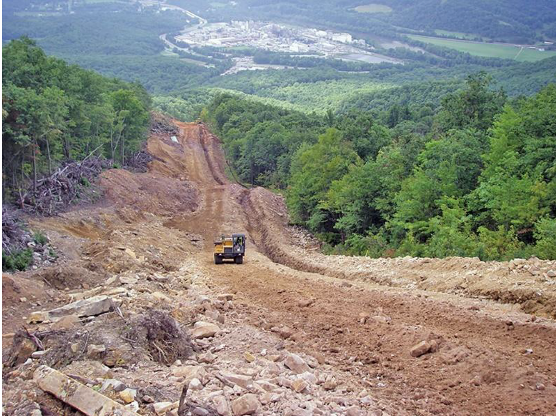
Figure 1.5.2 - Pipeline ROW under construction (Goodale, 2018). Impacts in this construction zone are extensive.
